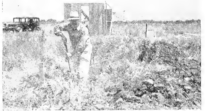
This is the beginning. I felt safer on the ground digging than I would on the tower.
